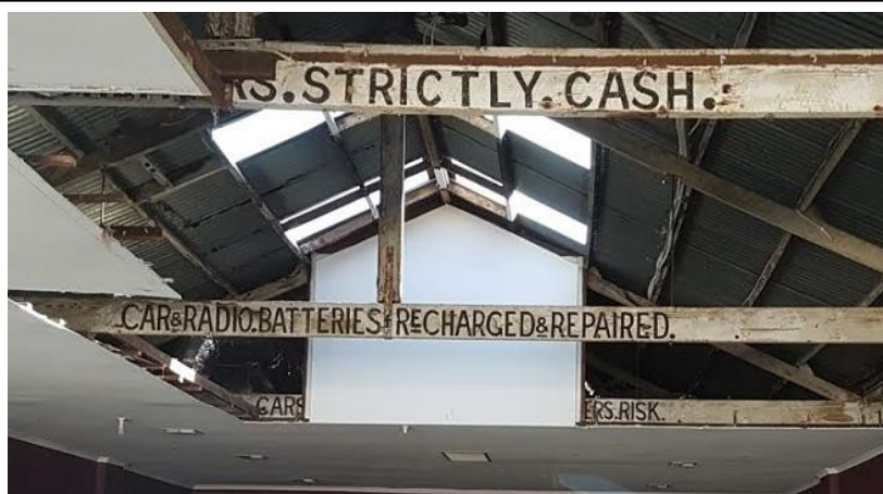
Renovations for a medical clinic in Nicholson Street in 2019 uncovered this signage that dates back to the days of Taggart Brothers' motor garage. (Image: CCHG)
